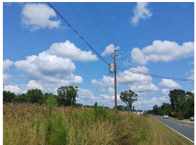
4: Eastern boundary of property and pole-mounted transformer, facing northeast along Harrill Road.
