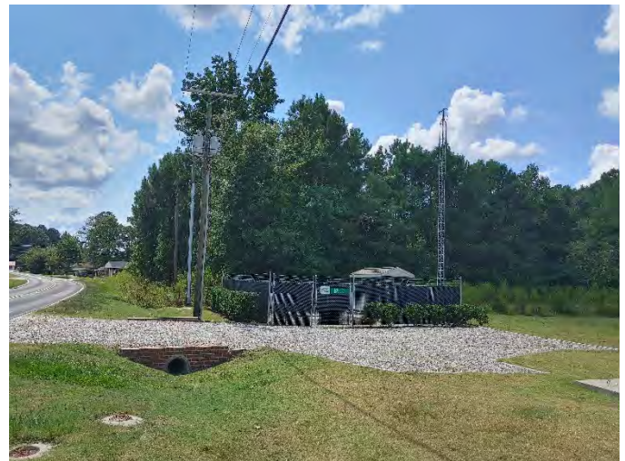
18: Northeast Pointe Liftstation #61 on adjacent property to the SW, facing south along Harrill Road.
