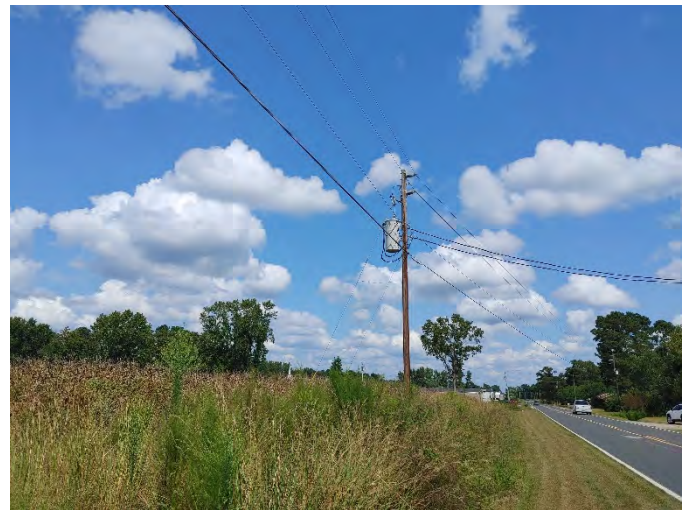
4: Eastern boundary of property and pole-mounted transformer, facing northeast along Harrill Road.
