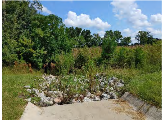
8: Retention pond overflows toward drainage ditch that runs along southwestern boundary of property.
